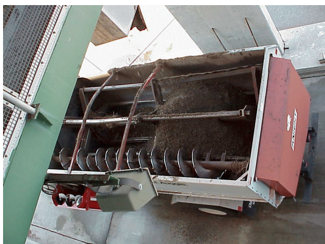
Picture 3. Academy Creek Wastewater Facility, Glynn County.
