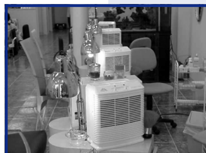
Individual charcoal air purifiers located at each nail care workstation
