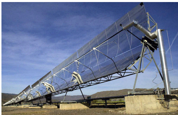
Figure 3. View of the PSA DISS solar field in operation
